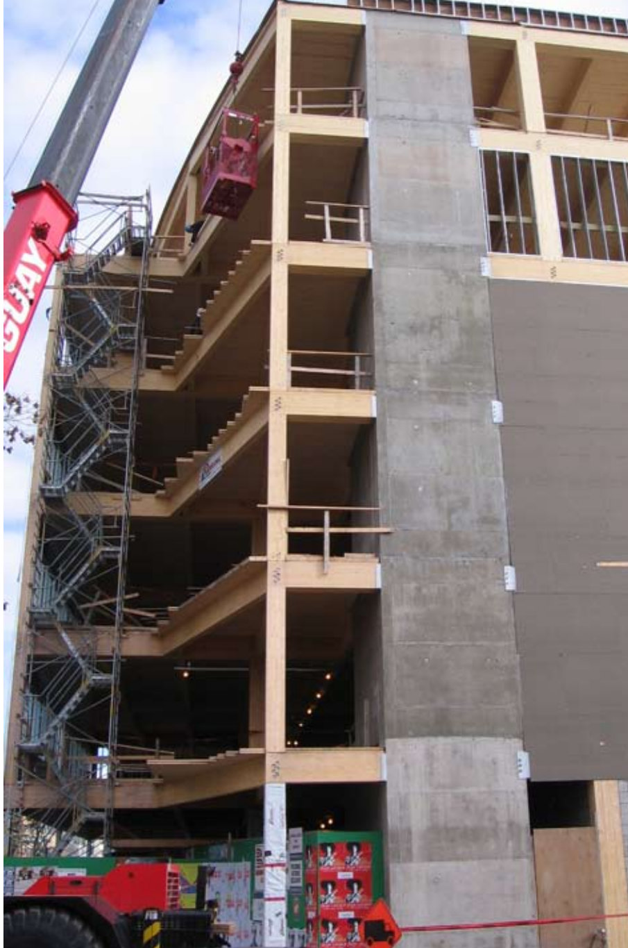
A six-storey glulam post-and-beam structure with reinforced concrete cores (CSN FondAction building) in Quebec City, Canada, illustrates how wood products can be used with other materials.
